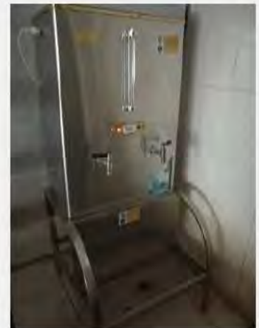
Drink water boiler
